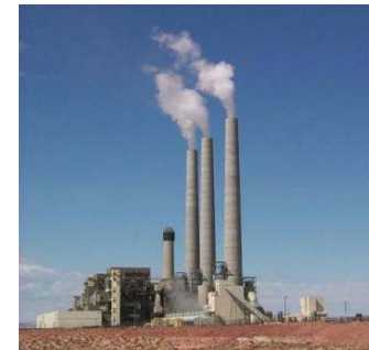
Power Generation from Waste Heat
