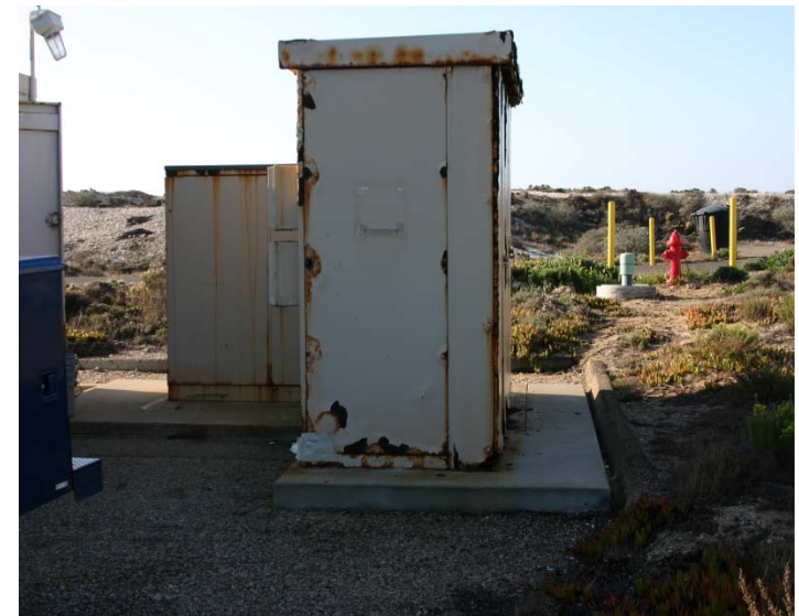
Sever Coastal Corrosion of conventional metal shelters
